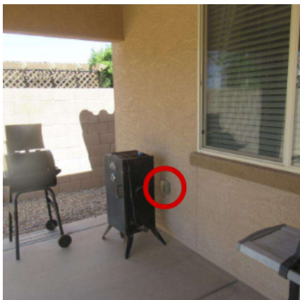
Image 3.3.1 Broken GFCI Location
