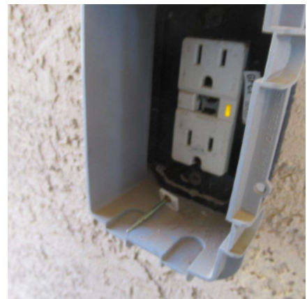
Image 3.3.3 Broken GFCI Test Button
