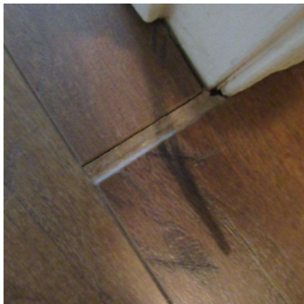
Image 6.1.1 Hardwood Flooring Gap - Master Bdrm Entry
