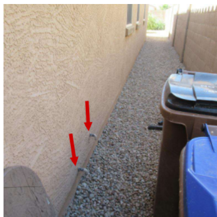
Image 5.1.1 Discharge Pipes on West Wall
