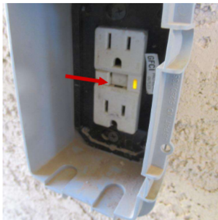
Image 3.3.2 Broken GFCI Test Button
