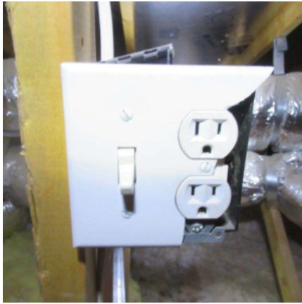
Image 3.4.1 Broken Outlet Cover
