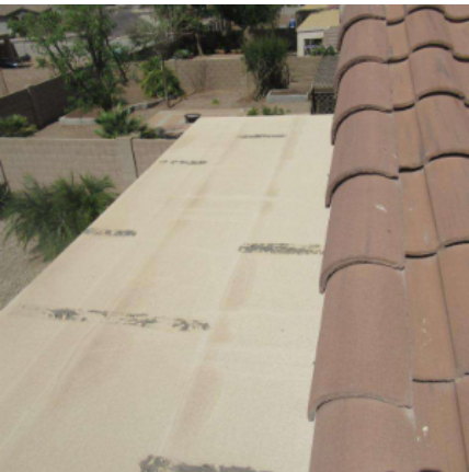
Image 2.2.2 Peeling coating from joints on patio roof
